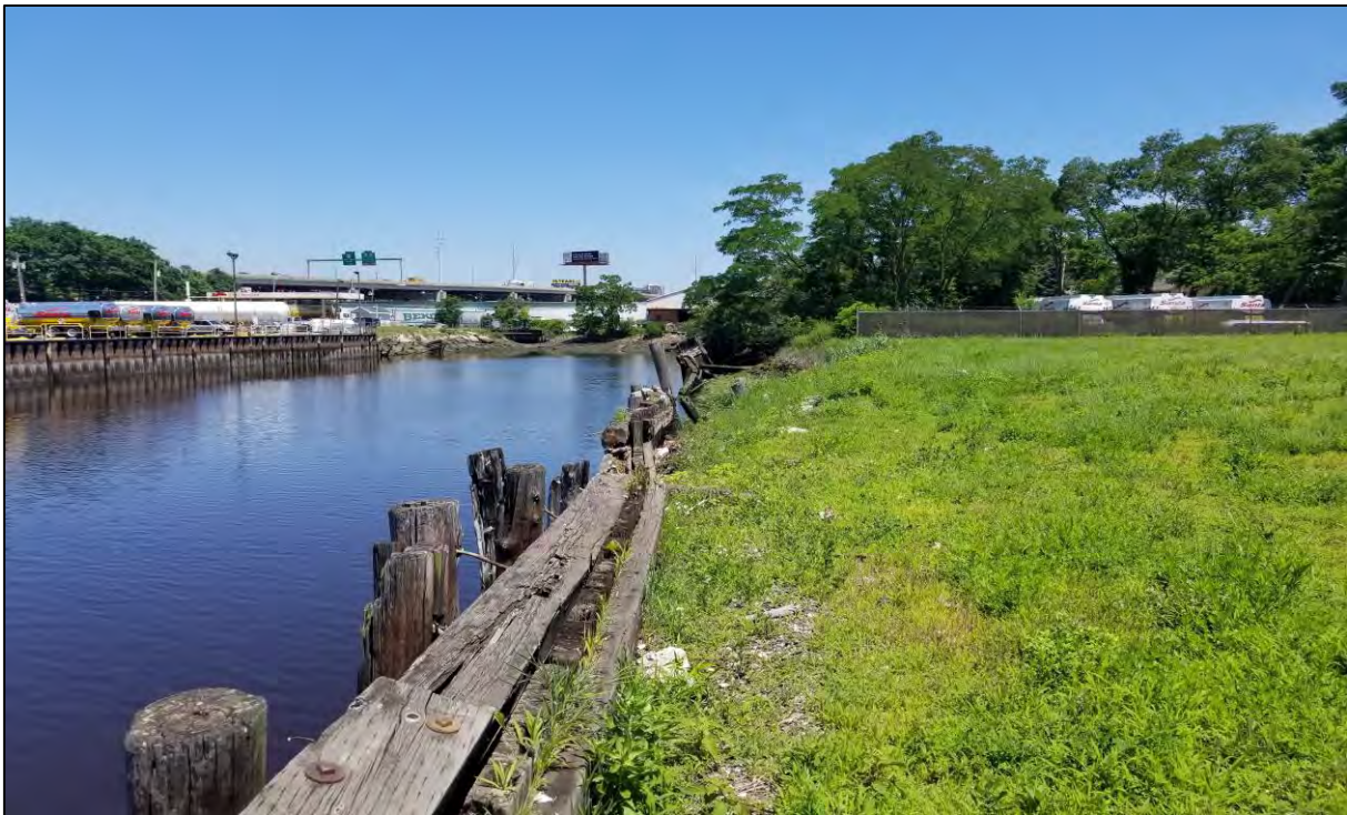
PHOTO 7: View of timber retaining wall along the approximate location of proposed Outfall E.
