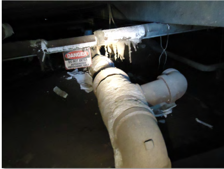
Photo 5: Potential asbestos containing pipe insulation in crawl space of apartment building.
