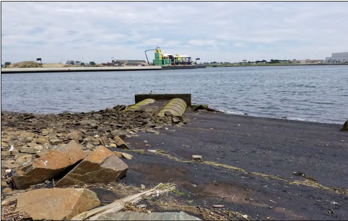
PHOTO 6: Existing Outfall D, looking east towards Bridgeport Harbor.
