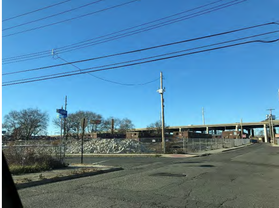
Northwest corner of Ridge Avenue and Columbia Street with an active construction site from building demolition within the RBD Pilot area beyond.
