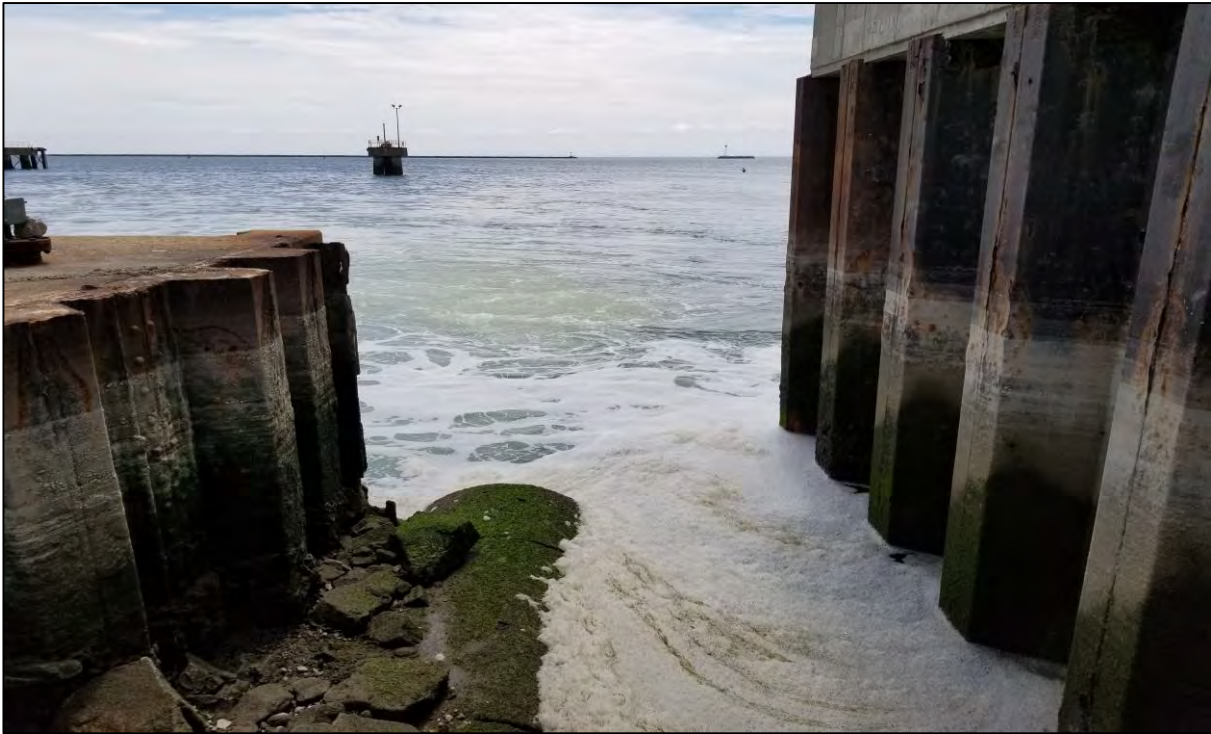
PHOTO 5: Existing Outfall C, partially submerged, looking south towards Bridgeport Harbor.
