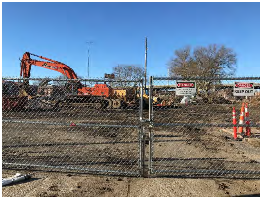
View of gated construction area entrance within the RBD Pilot area located along the approximate center of the north side of Ridge Avenue.
