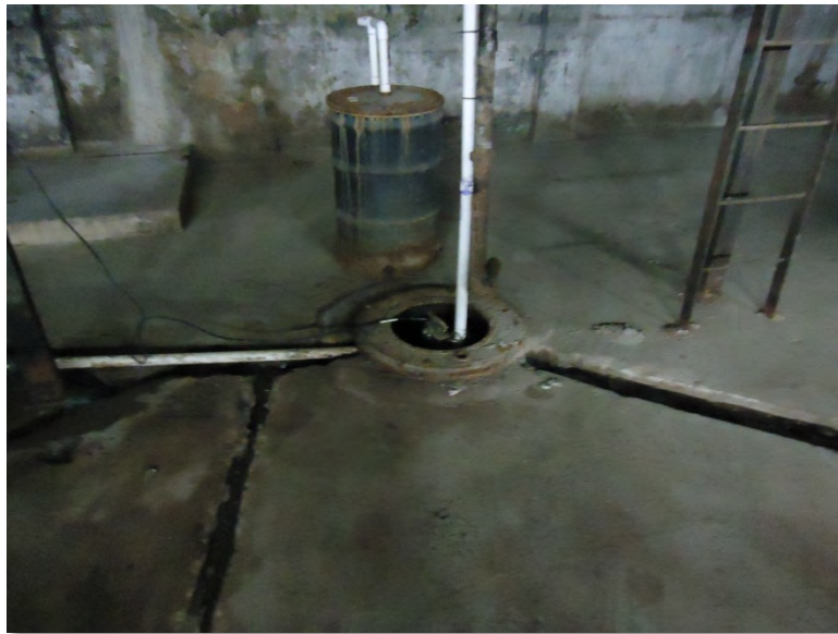
Photo 2: Sump pump in former boiler room in the Community/Maintenance Building.
