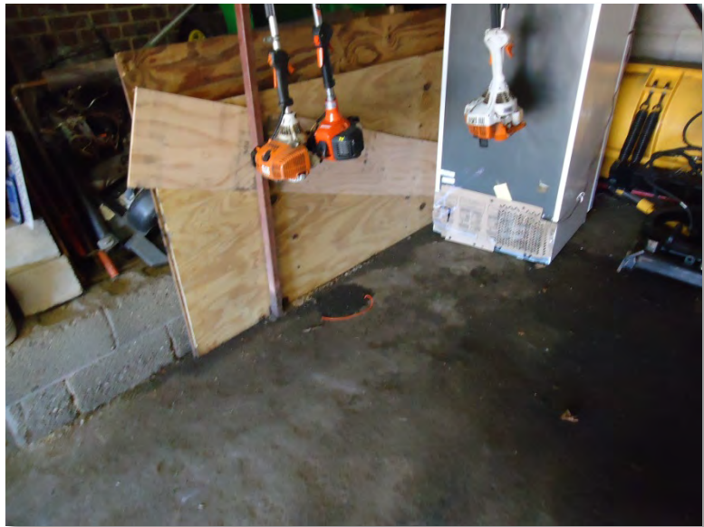
Photo 4: Minor staining below lawn equipment in the maintenance garage.
