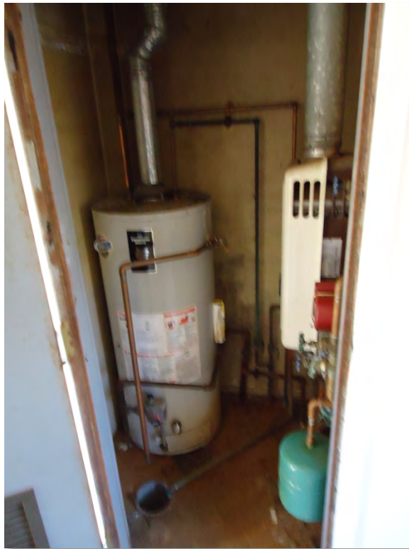
Photo 6: Furnace and hot water heater (both natural gas) in apartment unit.
