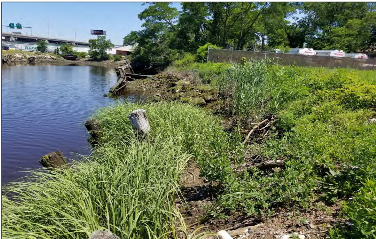
PHOTO 8: View of tidal vegetation ( S. alterniflora , Iva frutescens , Baccharis halmifolia ) along the collapsed portion of the timber retaining wall in the vicinity of proposed Outfall E.
