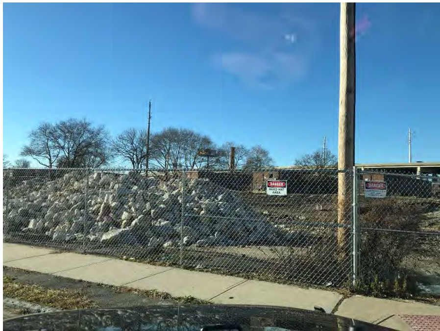
Zoom view of previous photo showing soil covered grounds, building demolition piles and buildings 15, 16 and 17 of the Marina Village Housing Complex beyond to the northwest.
