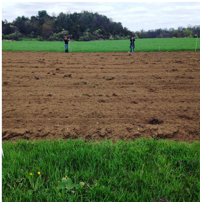
Installation of deer fencing at Sub Edge Farm in Farmington, CT to protect a field recently brought into production with financial assistance provided by the DoAg Farmland Restoration Program.
