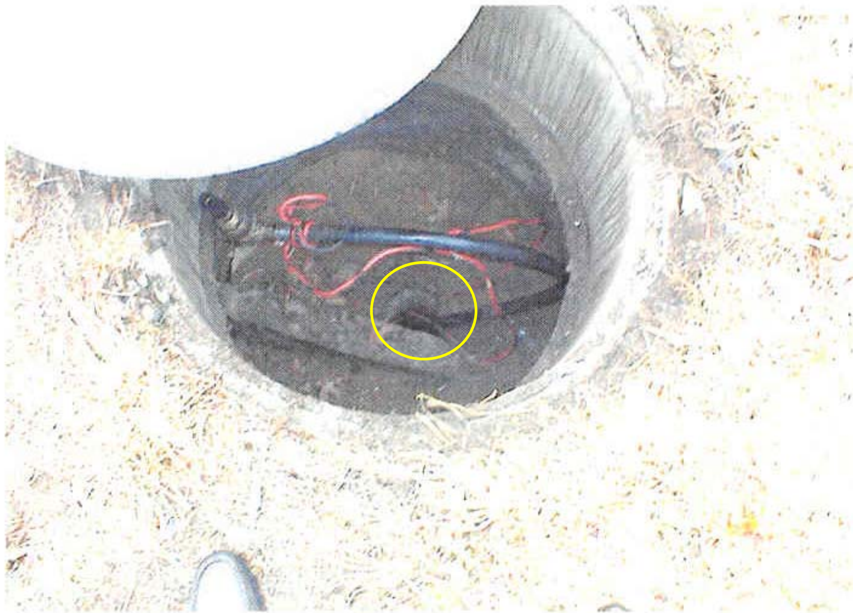
Pond View Apts.-Plainfield Well #1 Disconnected New Case Well Case
