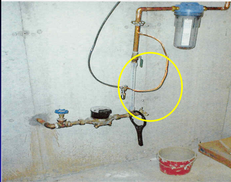
Disconnected Ground Wire 73 Cardinal Drive
