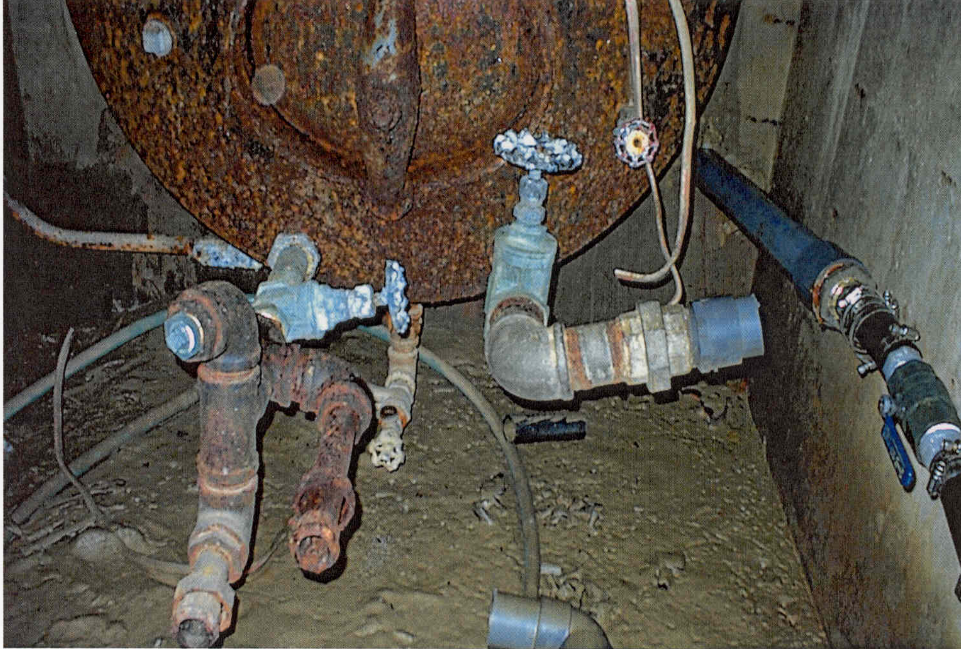
TANK DISCONNECTED WELL PIT SHOWS SIGH OF RECENT FLOODING
