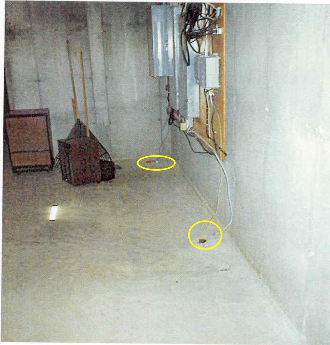
Double grounds in basement floor Monaco house
