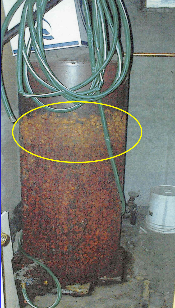
80-gallon Pressure Tank in 1 Building
