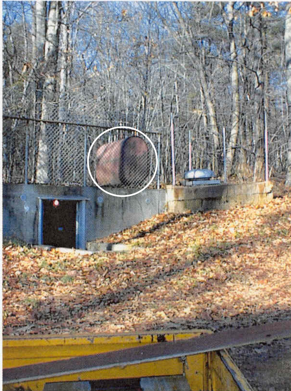
Pump house #1. Diesel fuel tank is located on top of the roof.
