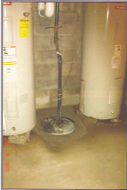
Photograph 3: Building 2, Unit 38 - Typical Basement Radon Proof Sump
