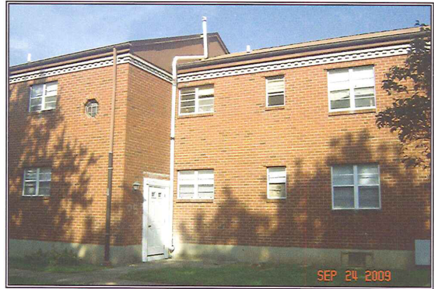
Photograph 9: Building 4, Unit 45 - Basement Venting System
