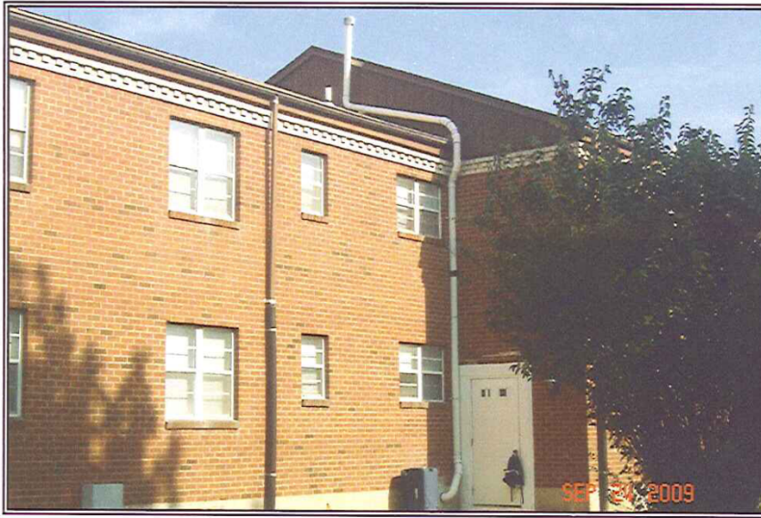
Photograph 8: Building 4, Unit 46 - Basement Venting System
