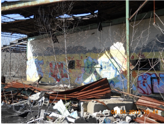
Collapsing Building, Debris Piles, Graffiti
