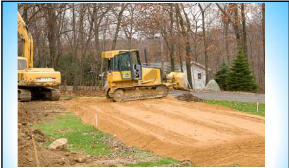
Fill must be compacted. A percolation test is required in the compacted fill if the leaching system is entirely within the select fill
