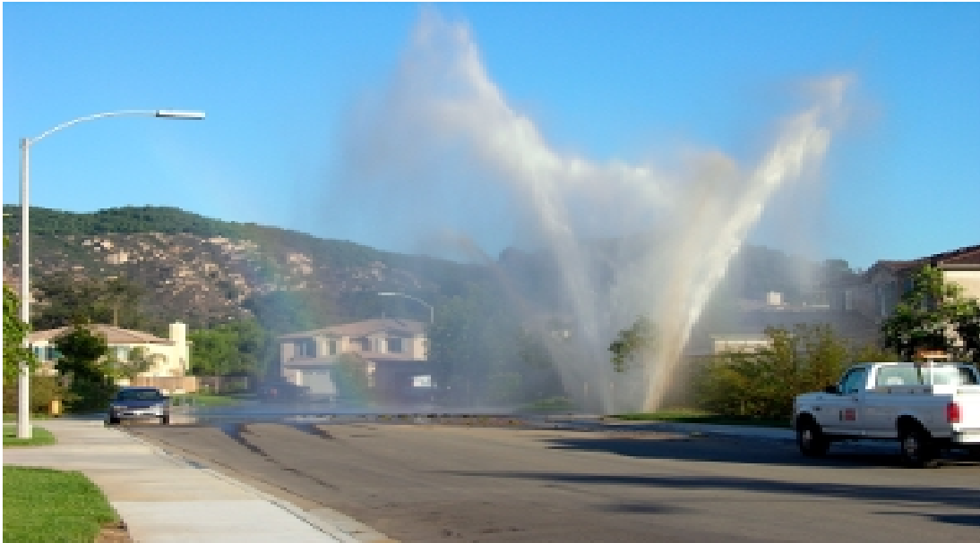
FIGURE 3-11. RUPTURE OF A 66-INCH WATER MAIN
