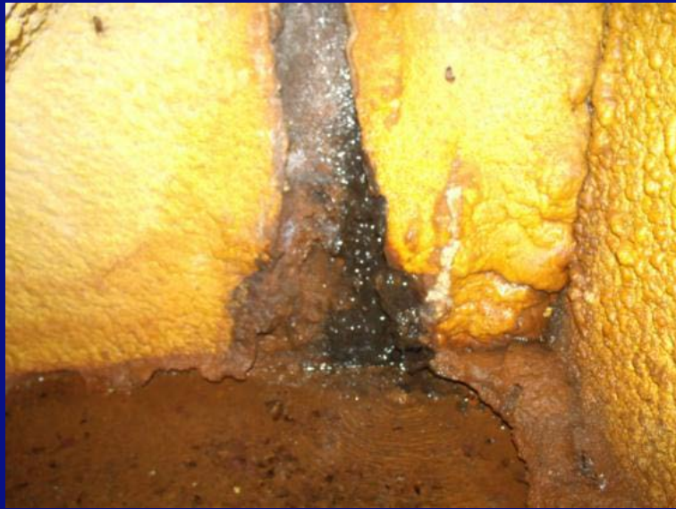
Foundation wall leaking water
