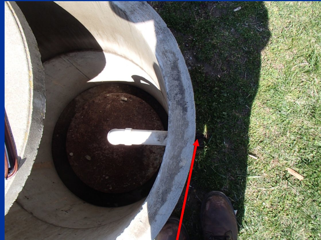
Vent/Overflow Pipe Broken
