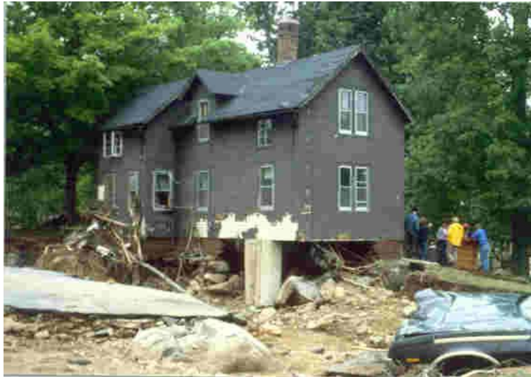
Figure 2-10: Downstream damage due to the 1982 Bushy Hill Pond Dam Break
