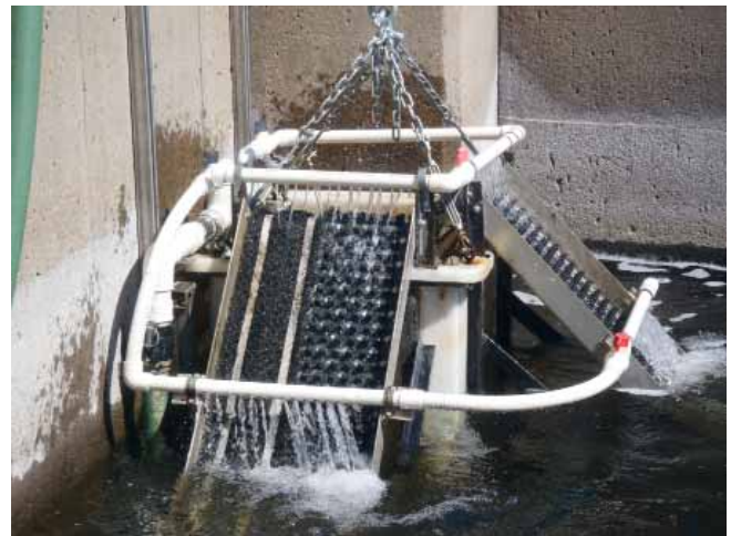
Believed to be the only eel lift in North America, the Greenville Dam Eel Lift is based on a lift design operating in New Zealand. While the basic concept between the two is similar, the eel lift is equipped with two short climbing ramps. It is unique because the whole apparatus is lifted upwards out of the water via an electric winch alongside a platform where staff can safely access the trap.
