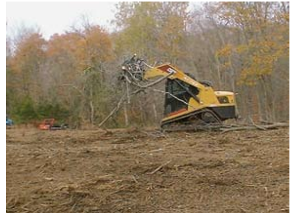
A fecon mower clears a field at Pease Brook WMA (Lebanon). The site, which was dominated by non-native invasive plants, is being converted to a warm season grass field.
