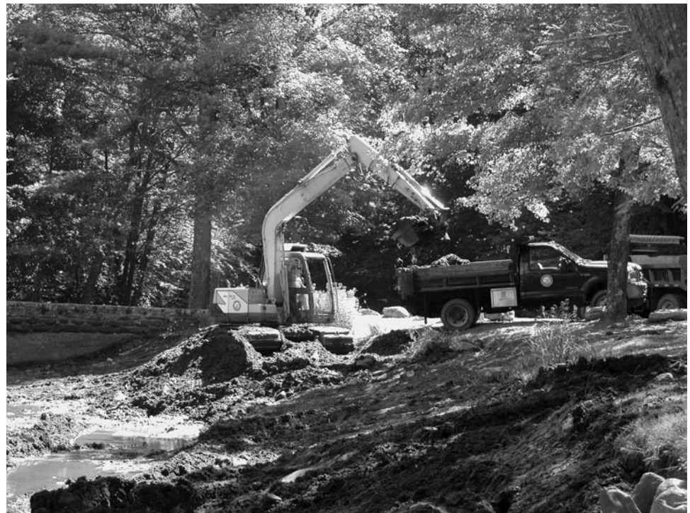
Using a low ground pressure excavator, the WHAMM Program assisted Chatfield Hollow State Park by dredging sediments from the pond, which is stocked with trout and open to the public.
