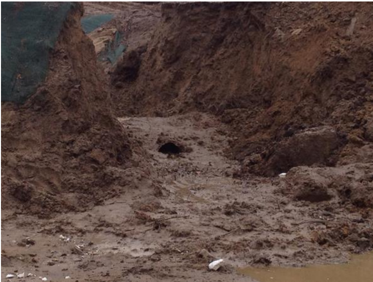
Figure 2 - Failure of Stormwater Basin Berm
