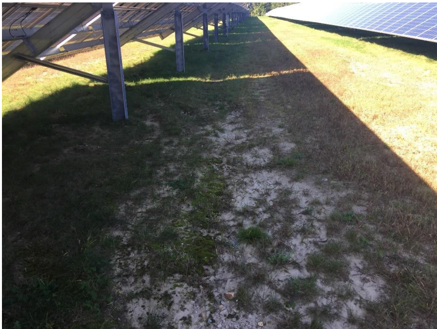
Figure 2 - Erosion & Sedimentation resulting from concentrated flow
