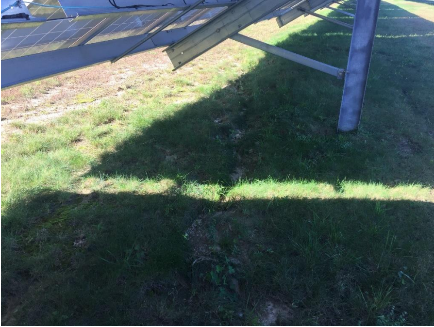
Figure 6 - Concentrated flow from runoff off solar panel
