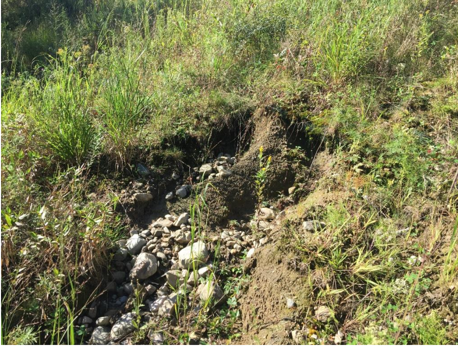
Figure 8 - Erosion of stormwater basin slope from concentrated runoff
