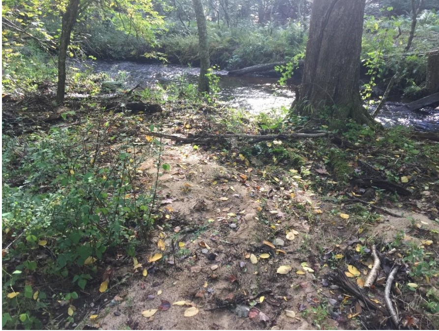
Figure 12 - Eroded material deposited adjacent to Cranberry Meadow Brook on Bialowans Property
