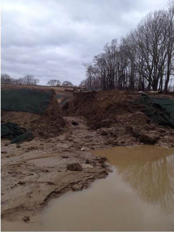
Figure 3 - Failure of Stormwater Basin Berm
