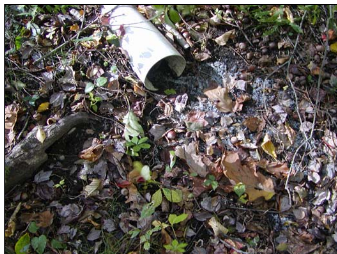
Figure 12: Fungal growth associated with the 6" PVC pipe discharging near the unnamed stream.
