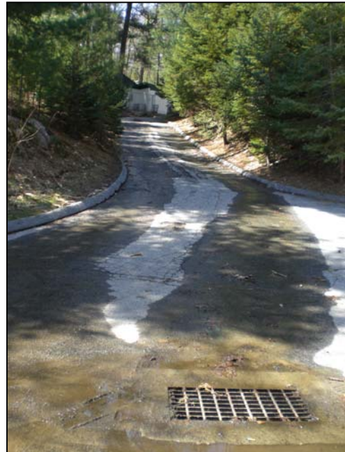
Figure 13: Overland Flow from the Animal Control Facility to a Storm Drain at the Maintenance Garage.
