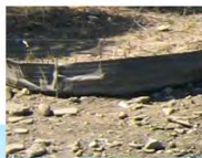
Failed Erosion Control
