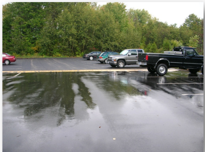
Porous pavement (top) in a lot beside conventional asphalt (bottom) at the UNH Stormwater Center (UNHSC) at University of New Hampshire.
