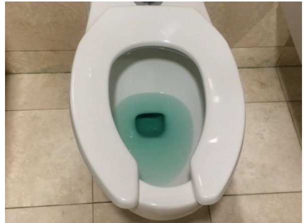
recycled water dyed blue being used for toilet flush
