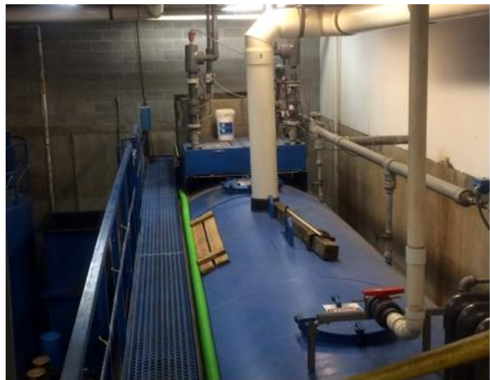
membrane filtration alternative treatment system
