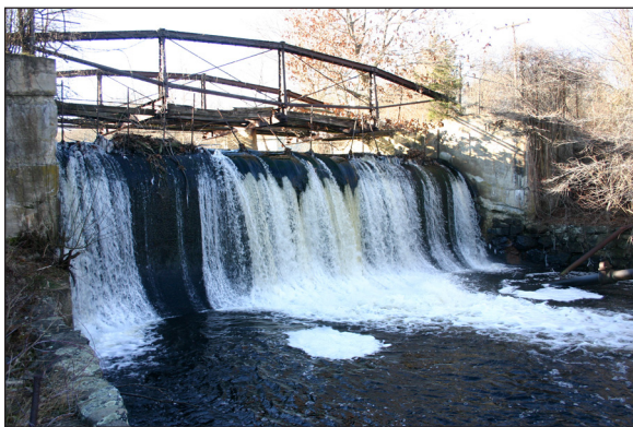
Hallville Dam, Preston, CT. A fish ladder will be constructed at the far right end of the dam.
