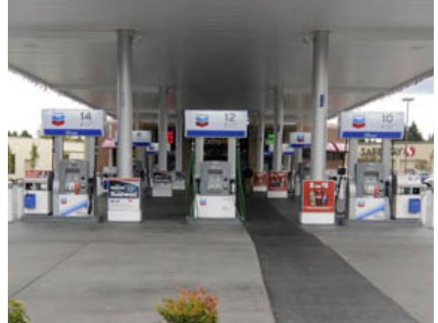
IMAGE 6. BEAVERTON, OR THE EVSE IS INTEGRATED INTO EXISTING INFRASTRUCTURE. IT IS LOCATED BETWEEN OTHER GAS PUMPS AS TO NOT BLOCK TRAFFIC SINCE THE CHARGING VEHICLE MAY BE PARKED FOR UP TO HALF AN HOUR.
