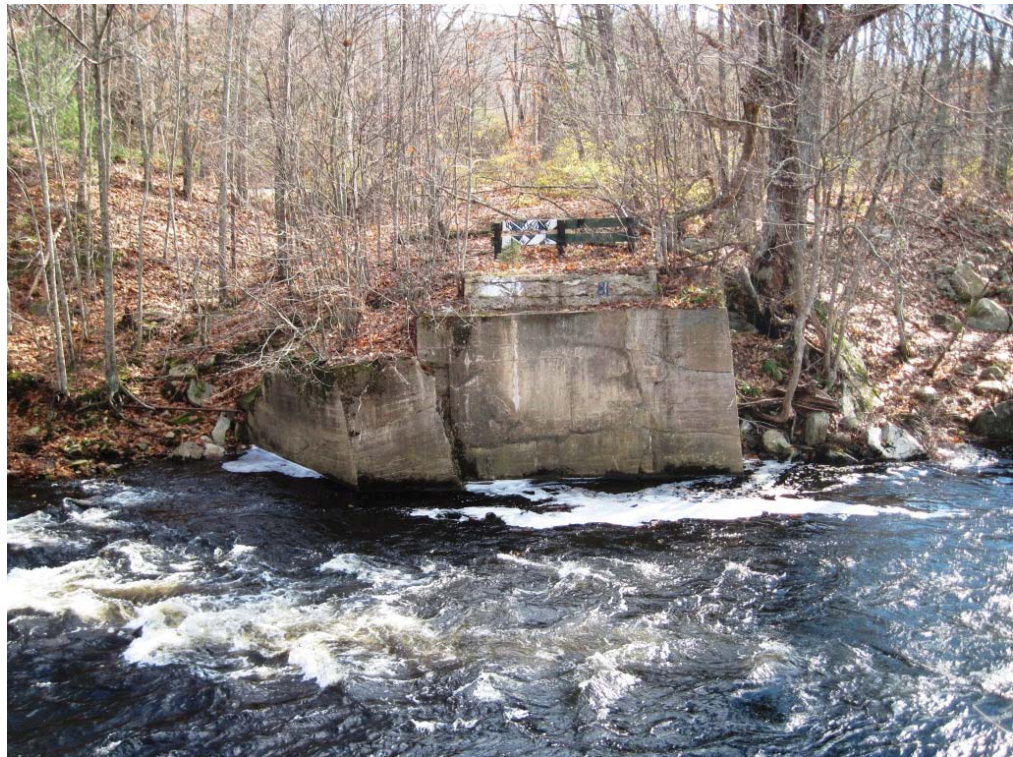
Pipeline Segment 12B: Former Bridge Abutment in Mansfield Viewed from Jones Crossing Road
