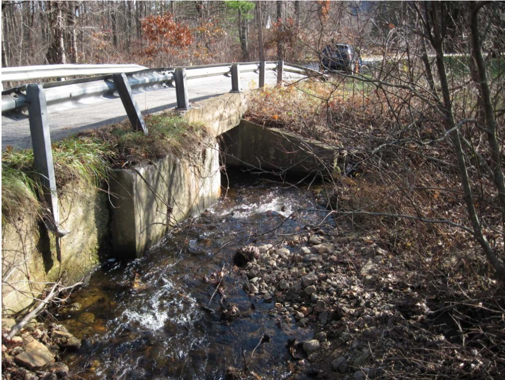
Pipeline Segment 12B: Clark Brook Box Culvert on Jones Crossing Road (Coventry)
