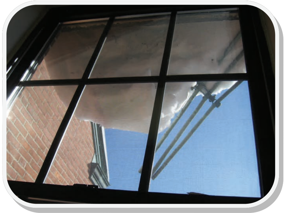
Large amounts of snow sliding down the roof of Jones Auditorium in New Haven. This chunk tore off part of the snow guard. Photo by Katherine Dugas.
