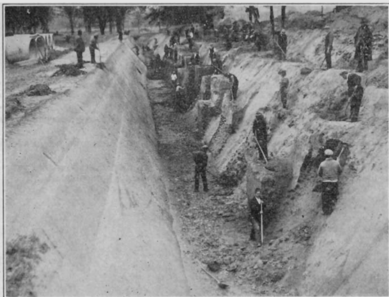
FIGURE 96. Laborers excavating a deep main ditch from East Hartford meadows to Connecticut River.
