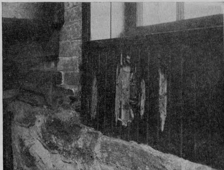
FIGURE 125. View near basement stairway of the Union Town Library, showing damage to the wainscoting by white ants.
